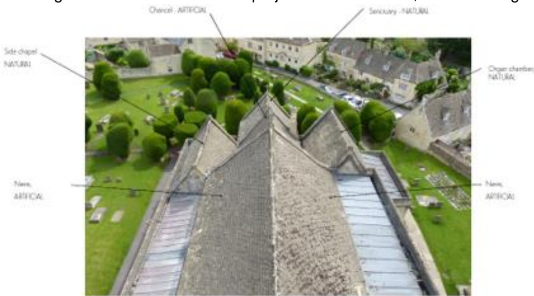
Before: Photograph showing the roofs to be replaced alongside the existing Cotswold Stone roofs
