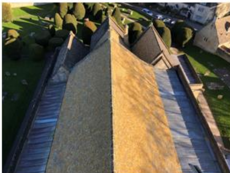
After: Photograph showing the roofs on completion of the project: all roofs of natural Cotswold Stone
